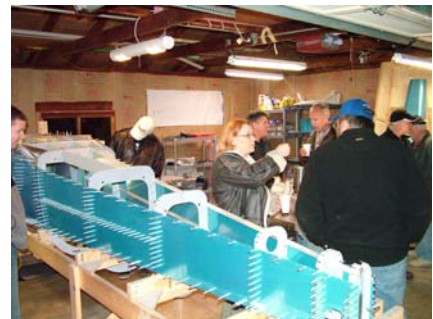
The underside of the fuselage, bristling with clecoes is seen in the foreground as folks like Gwen talk shop.
